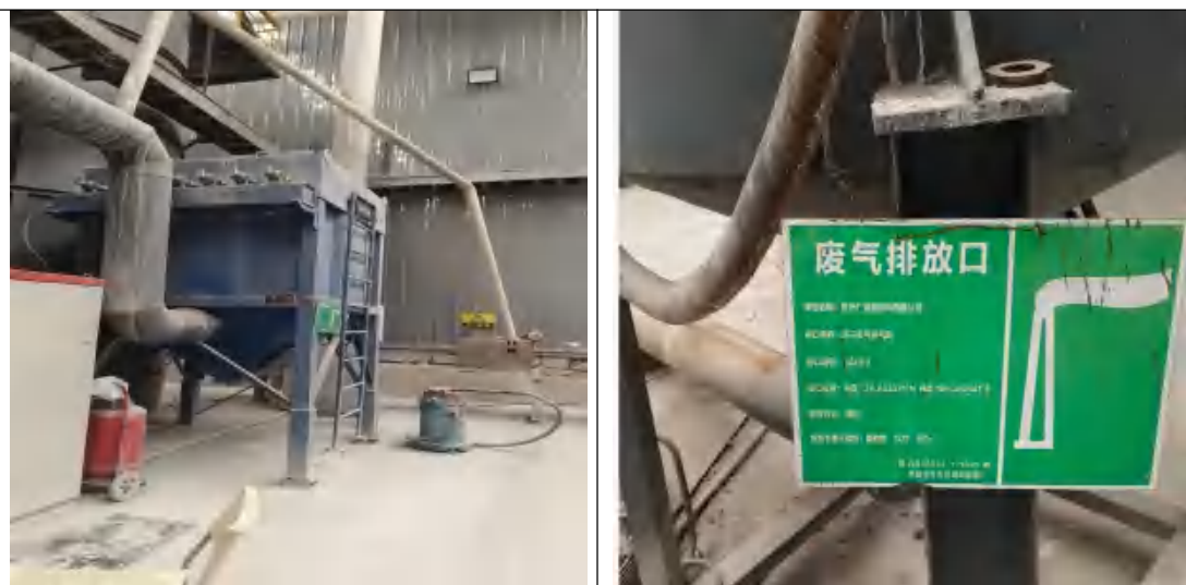
烘干机废气排气筒
